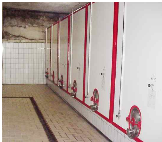
Concrete tanks for the fermentation of wines
